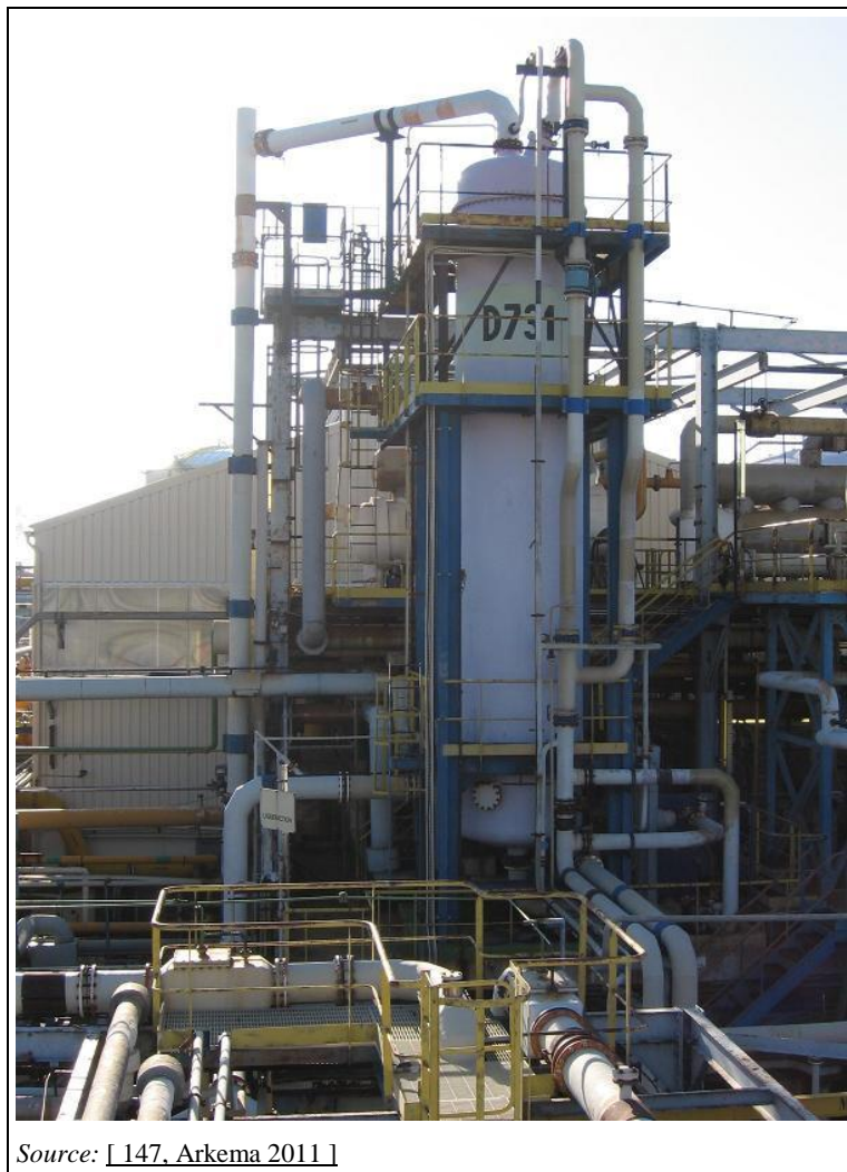
Figure 2.18: View of a chlorine absorption unit
