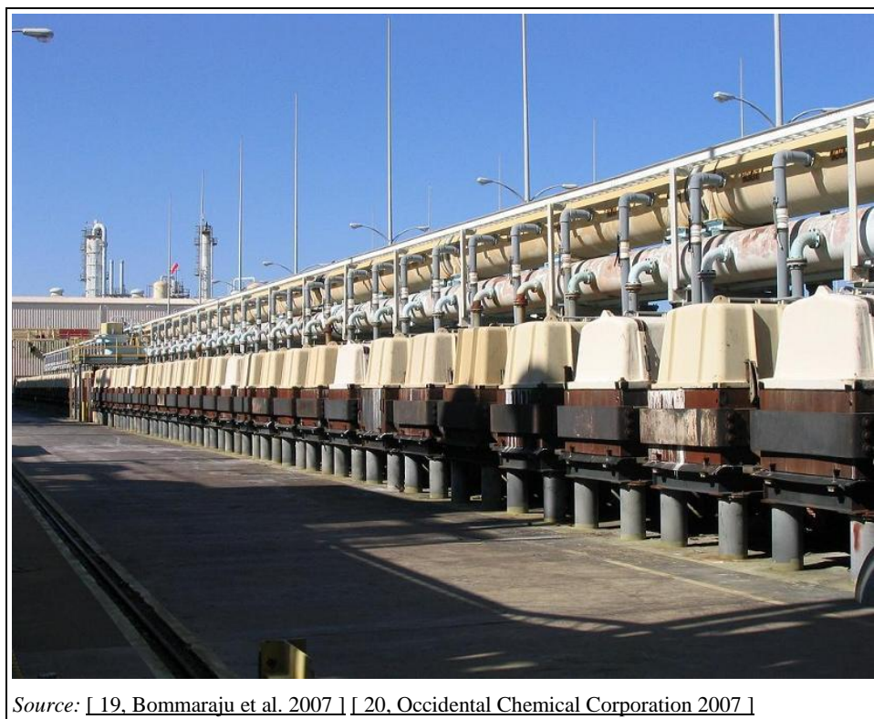
Figure 2.7: View of an open-air diaphragm cell room equipped with monopolar electrolyzers
