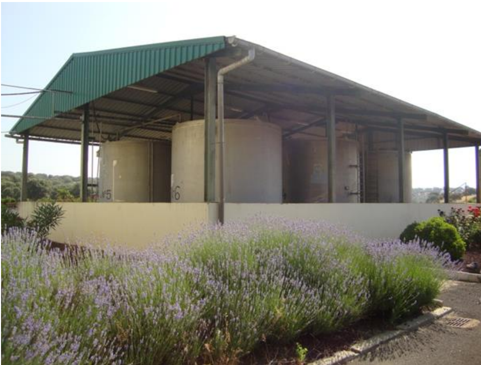
Mercury storage tanks (6 tanks of 30 m 3 of capacity each).
